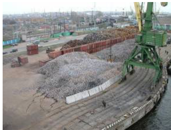
Figure 2 – Deformation of the berth due to overloading
