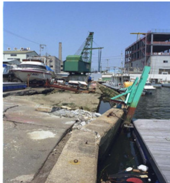
Figure 5 – Deformations of the berthing facility cordon line
