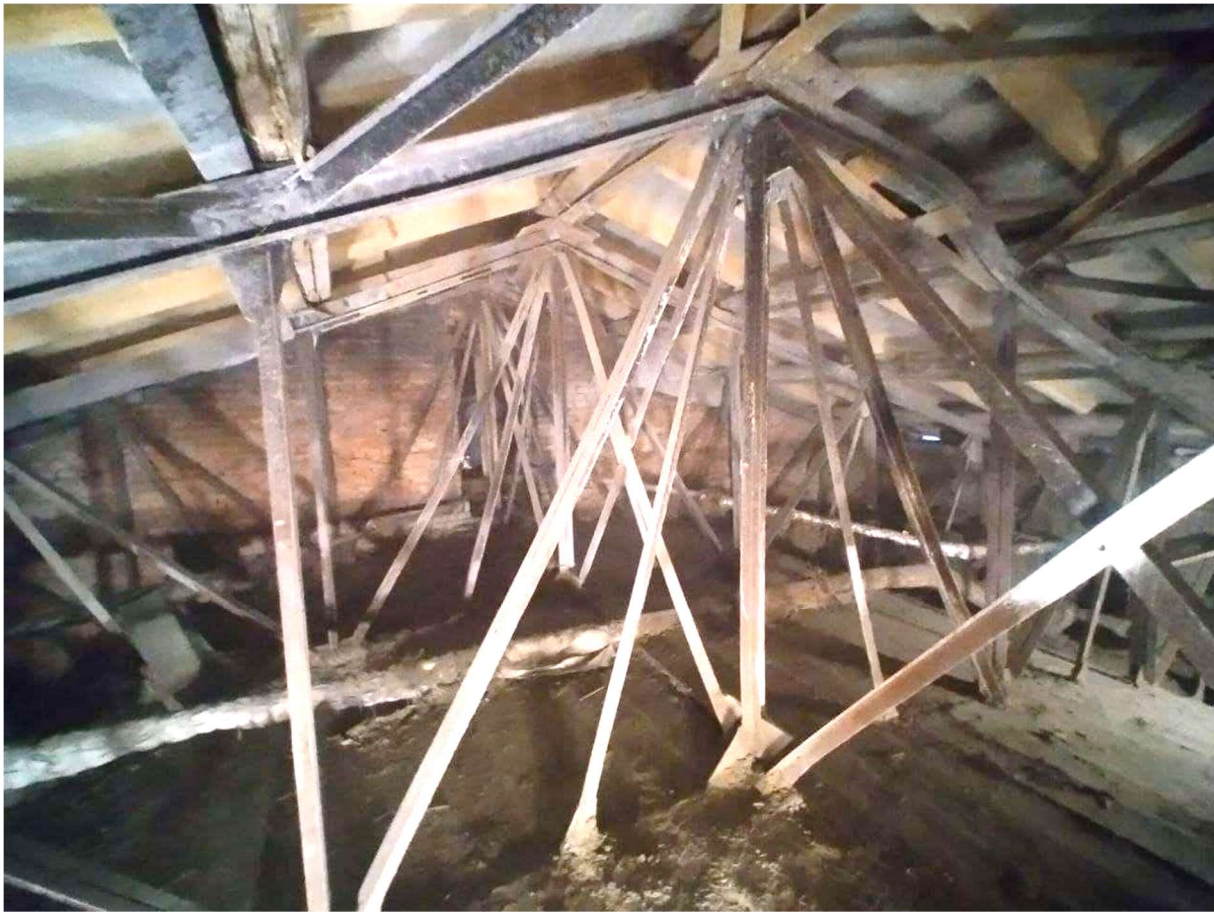
Figure 3 – General view of the steel structures of the roof of the hall at the time of the survey: ordinary load-bearing trusses of the concrete vault
